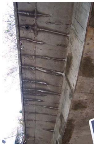
Fig. 16: Early thermal contraction cracks at underside of cantilever slab
