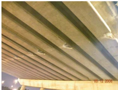
Fig. 2: Damage at underside of beams of a bridge in Shah Alam due to vehicular impact
