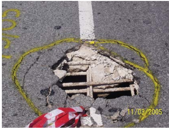
Fig. 8: Pot hole in the deck slab initiated by cracks similar to Fig. 21
