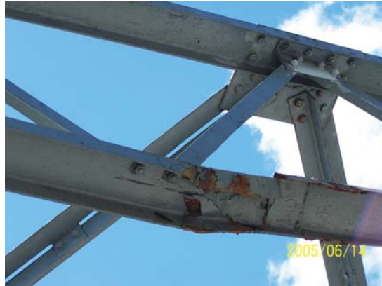
Fig. 20: Deformation of member of a steel truss bridge in Sarawak due to vehicular impact
