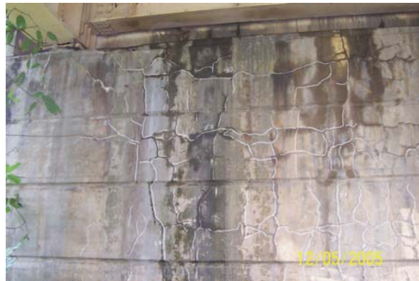
Fig. 17: Random map cracking (chalk line drawn alongside) at the abutment of Tamparuli Bridge resembling that of AAR
