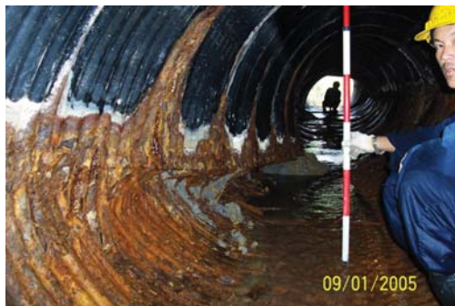
Fig. 22: Widespread corrosion at bottom half and joints of a CMP
