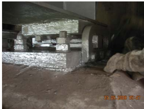
Fig. 28: Bolts and restraining frame of the bearing in the autopont bridge reinstated and painted
