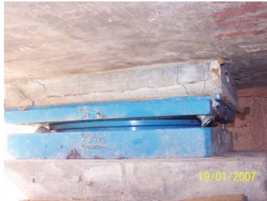
Fig. 29: Anchor bolts and plinth damaged
