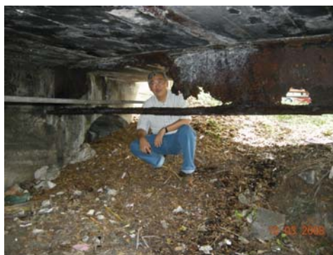
Fig. 19: Total loss of section of a steel girder bridge in Ipoh
