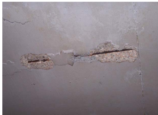
Fig. 12: Cracks and spalling of concrete due to carbonation
