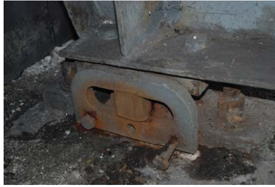
Fig. 27: Damaged mechanical bearing of the autopont
