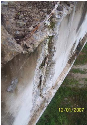
Fig. 30: Crushed parapet at the expansion joint due to movement of the deck
