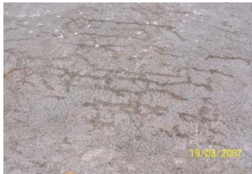
Fig. 15: Plastic shrinkage cracks on top of the deck slab
