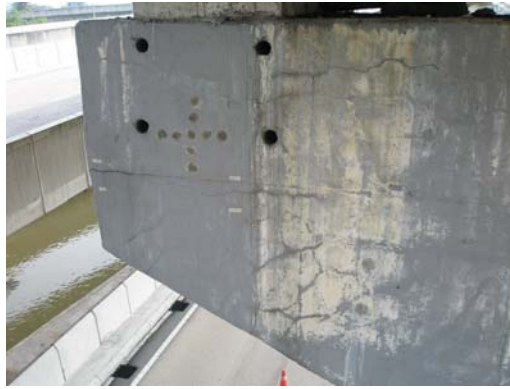
Fig. 18: Multiple cracks of a bridge pier in K.L. that was caused by DEF
