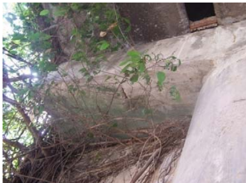
Fig. 3: Vegetation growth at bridge abutment
