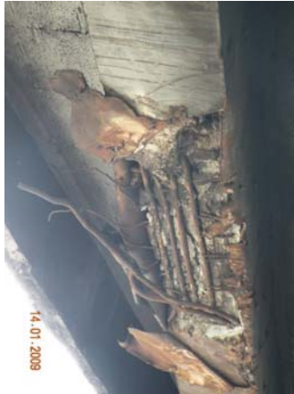
Fig. 1: Damage at underside of a beam in K.L. due to vehicular impact
