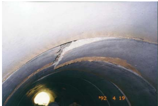
Fig. 6: Flexural problem in RC culvert (note tension crack at the crown)
