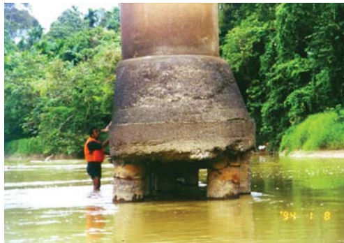
Fig. 32: General scouring of river bed at Sg. Jeniang
