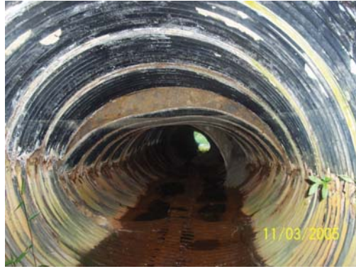
Fig. 23: Failure of CMP due to loading
