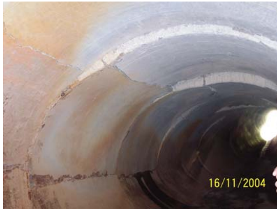
Fig. 7: Flexural problem in RC culvert (note compression crack at mid way of the wall)
