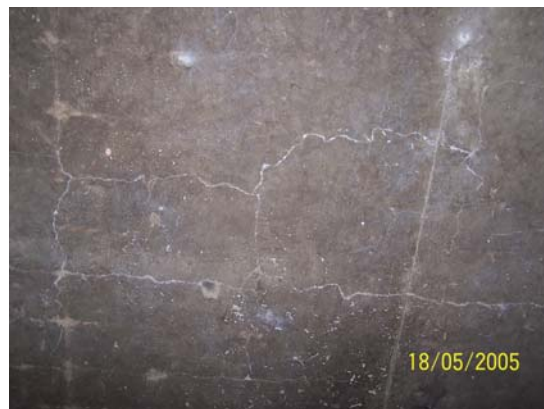
Fig. 21: Cracking at the underside of concrete deck slab of a steel truss bridge
