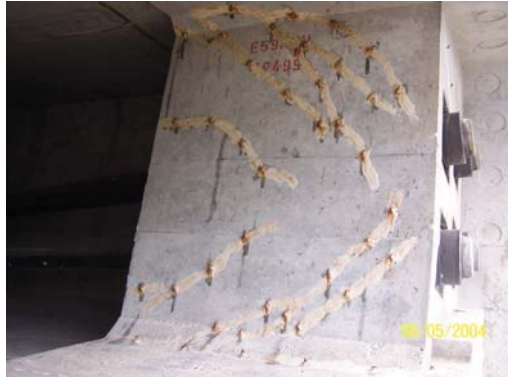
Fig. 11: Cracks at the anchorage zone (sealed with epoxy) of a box girder
