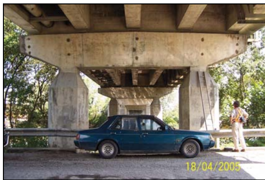
Fig. 9: Cracks in the reinforced concrete bent caps
