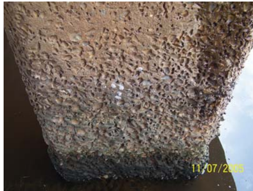
Fig. 4: Acid attack of lime stone aggregates
